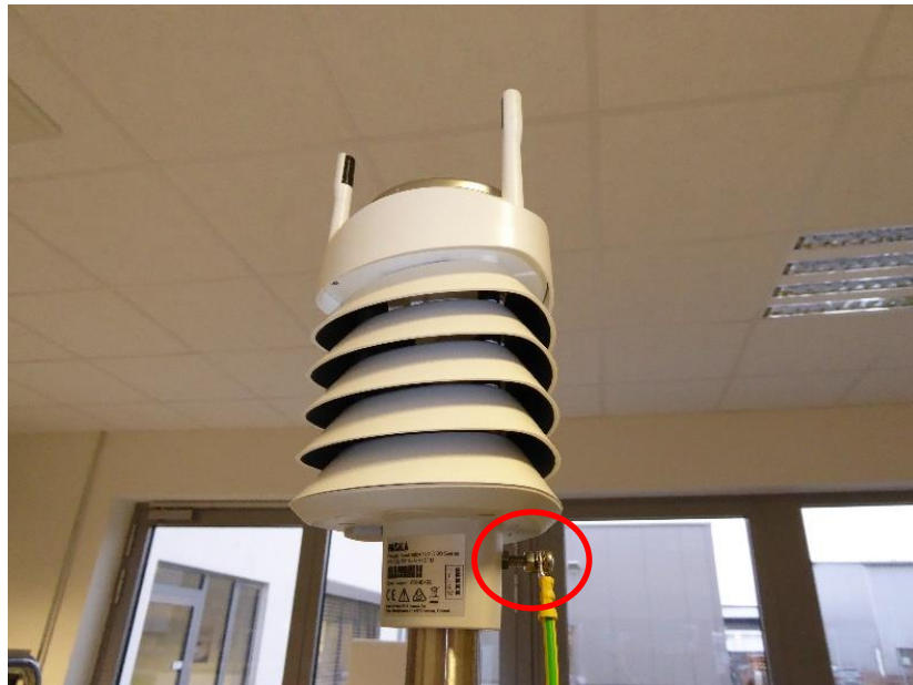
Grounding point on the weather station.
