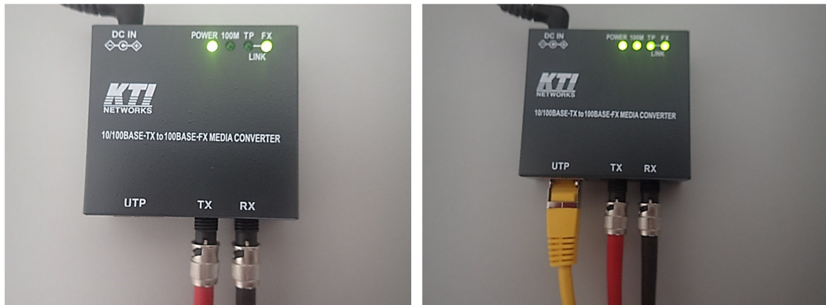
2 line fiber optics to LAN-TCP/IP converter.
