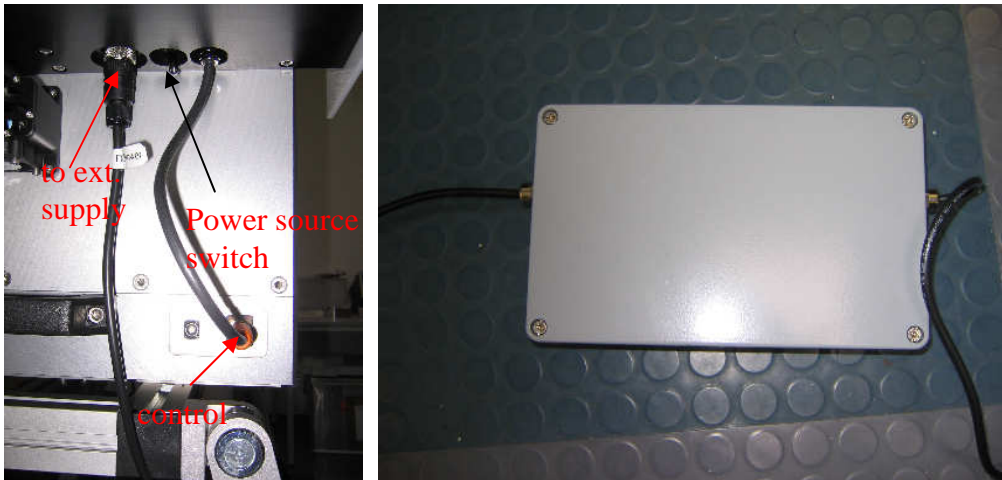
Fig.1.9: Electrical dew blower connections and external power supply.
