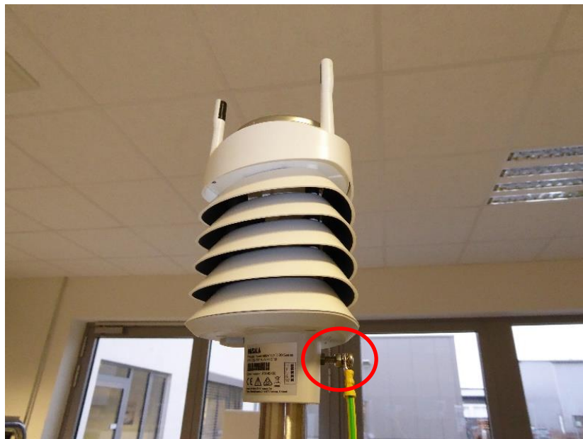
Grounding point on the weather station.
