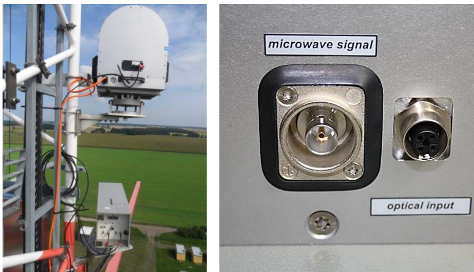
Figure 19: Left: OMS transmitters mounted on a measurement tower in Lindenberg, Germany. Right: BNC connector (left) to read the RPG-MWSC-160 detector voltage (only for diagnosis).
