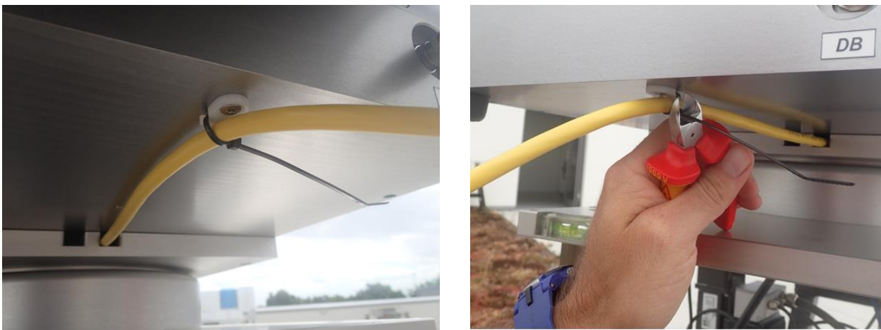
Fig.2.6.8: Fixing AC2 cable on radiometer bottom plate and cutting the cable tie.
